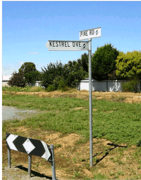
Photo 1 – Correct installation except for pointed end on Kestrel Drive sign.
