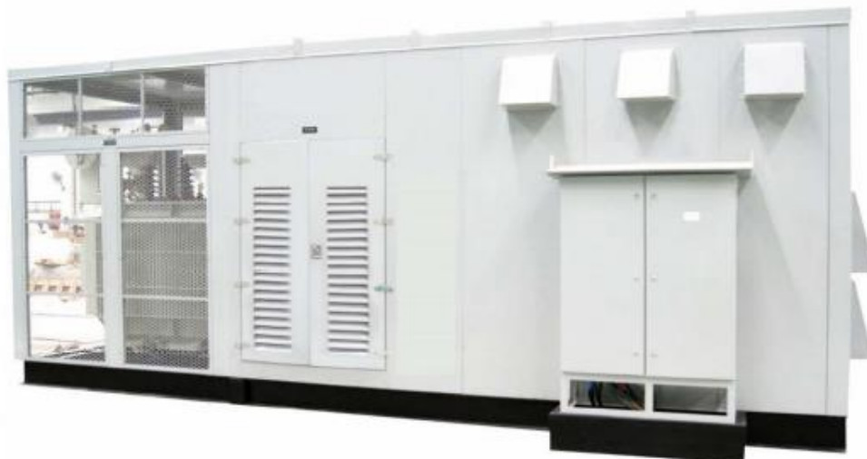
Figure 7 Example of a containerised photovoltaic box
