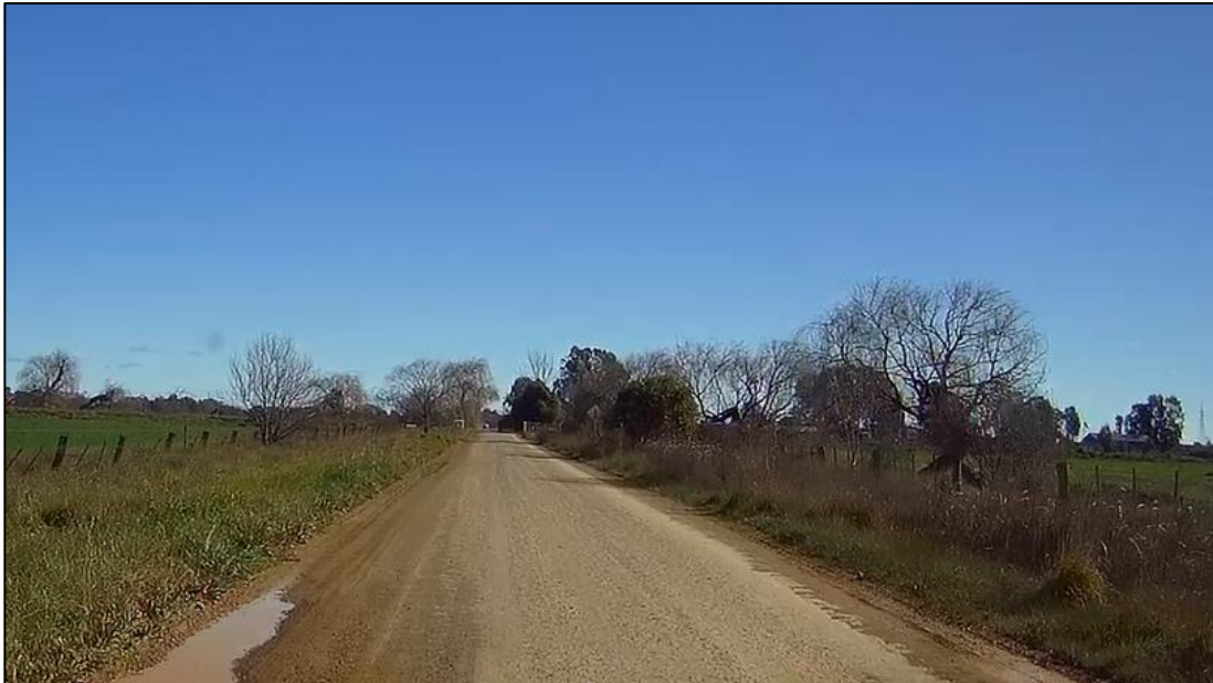
Photo 6: the unsealed section of Pyke Road, looking west near to the intersection with the Tatura-Undera Road
