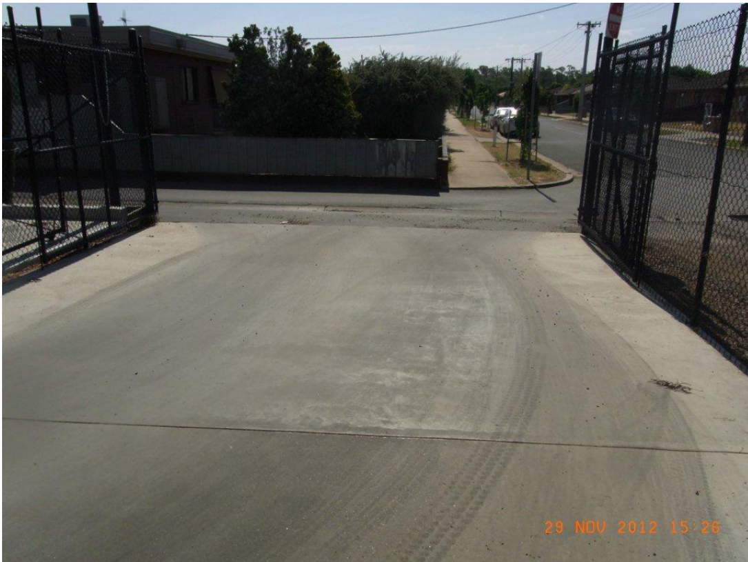
Intersection from the land to Bowe Lane and location of proposed speed hump
