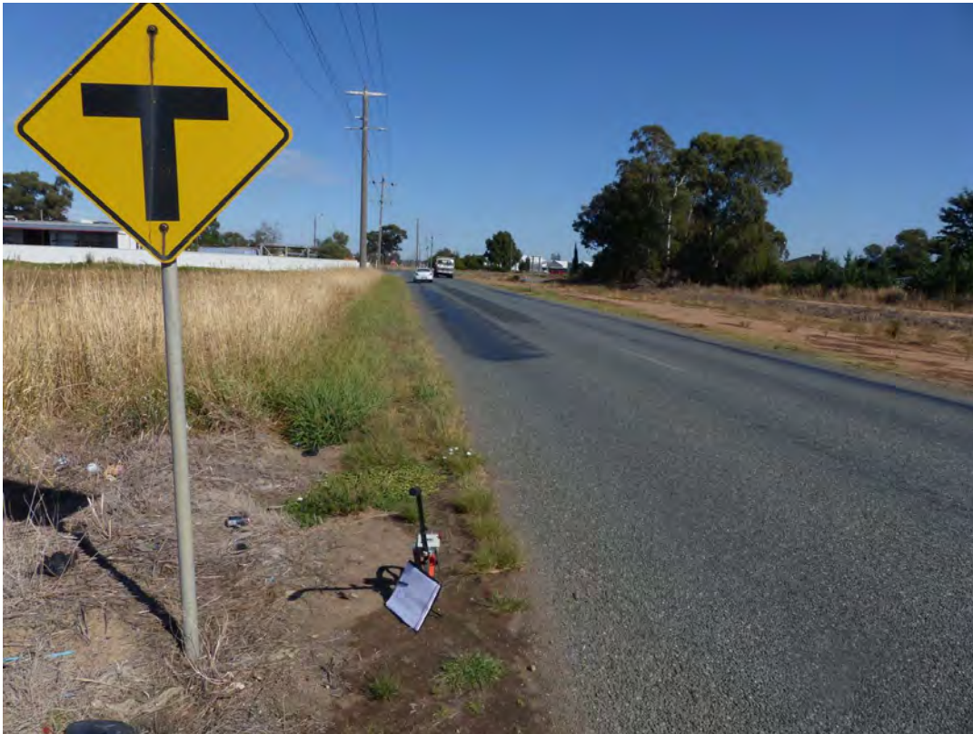
Photograph 3 Ford Road; view to west at Ch. 2500 approaching the GV Hwy; severe flushing in west-bound lane
