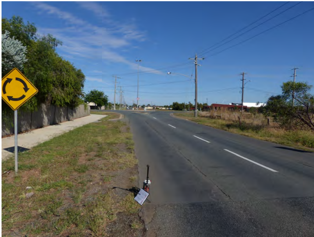
Photograph 2 Ford Road; view to west at Ch. 1380 on approach to Verney Road roundabout; widening pavement showing distress
