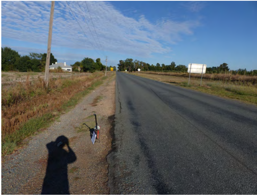
Photograph 1 Ford Road; general view to west at Ch. 100 3 ; pavement is in generally fair condition with some flushing in wheelpaths
