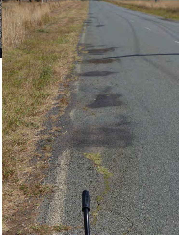
Photograph 8 Wanganui Road: Depressed edges with bleeding coming through the spray seal; Ch. 2000; view to east
