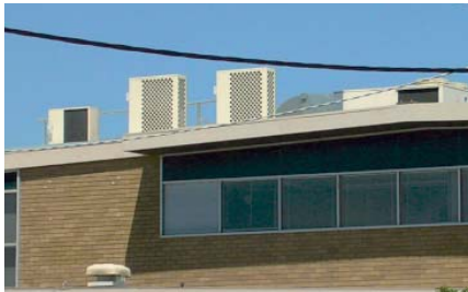
Plant equipment dominates the roofline and must be avoided.
