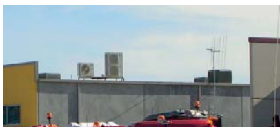
Roof top equipment should be integrated into the roof design so as to avoid its visibility from the street. X
