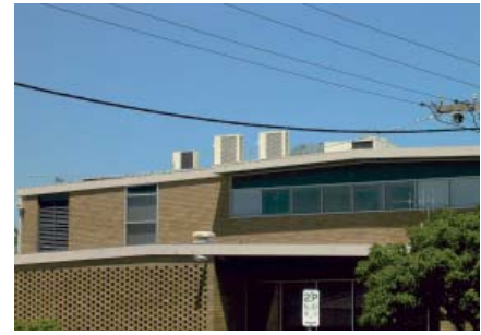
Roof top plant equipment
