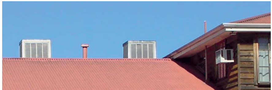
The roof top equipment on this building is visible from the street and must be avoided.
